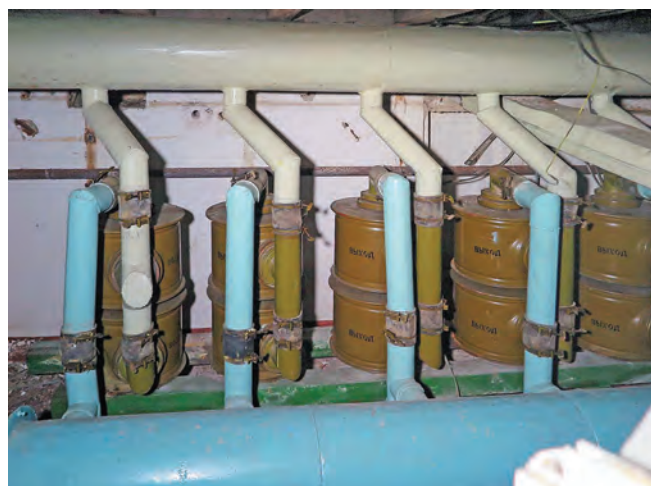
Soviet air filters bridge the colour coded external and internal air systems. Photo Clive Penfold
